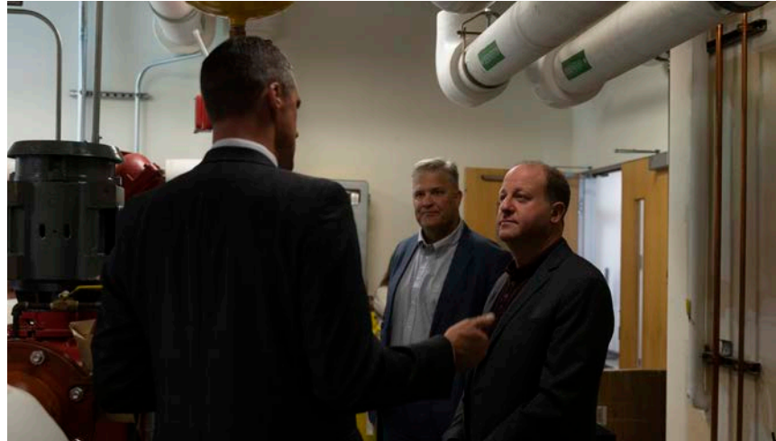
Governor Jared Polis toured the geo-exchange system at Colorado Mesa University (CMU) with University President John Marshall. With additional state funding approved by Governor Polis, CMU hopes to become the first university in the country to use geothermal energy to heat and cool 100 percent of its campus.
