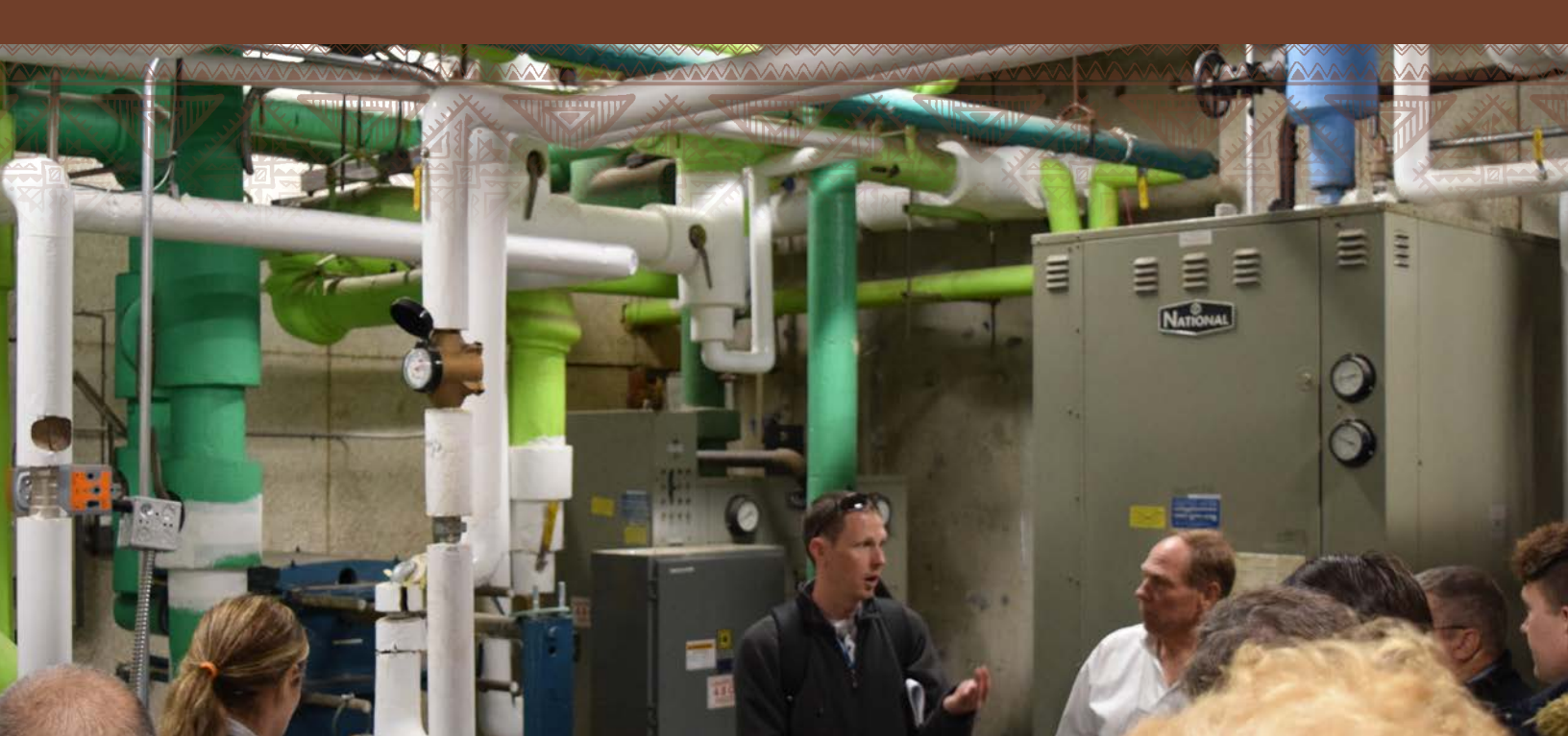
Jon Gunnerson, the Geothermal Coordinator for the City of Boise, explains to workshop participants how the Boise Warm Spring Water District has expanded operations from heating just a handful of buildings in 1892 to now sustainably heating 6 million square feet of building space.
