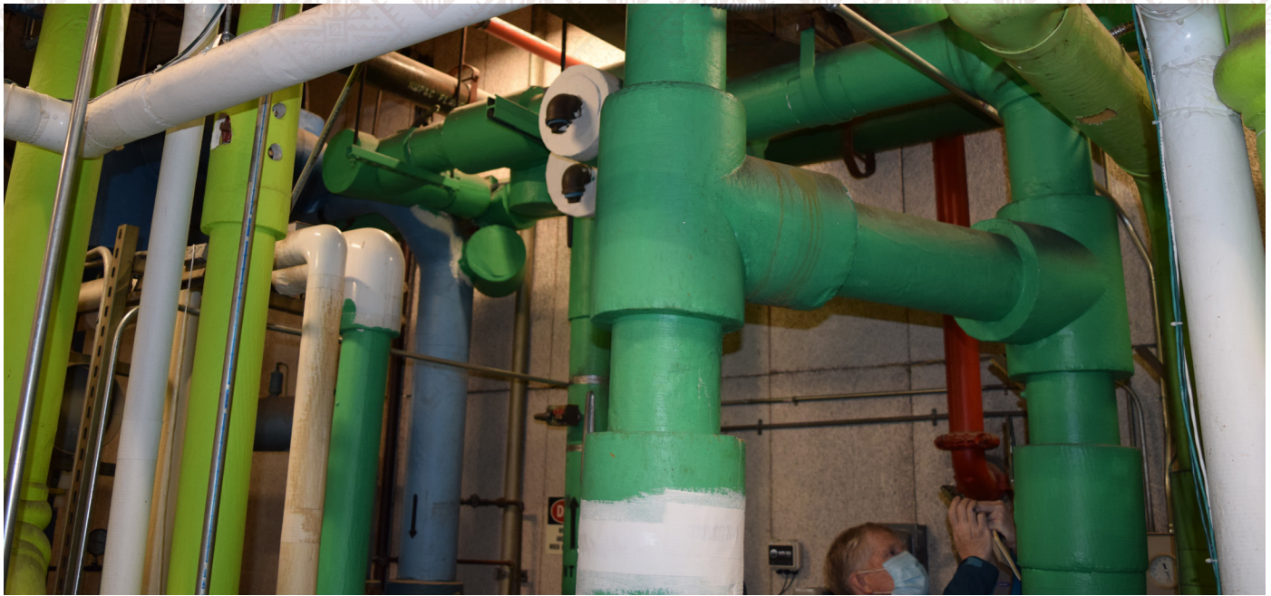
Beneath Boise's City Hall lies an intricate network of pipes that act as a heat exchanger for the city's geothermal district heating systems. Idaho workshop participants toured the mechanical room at City Hall to view the infrastructure.
