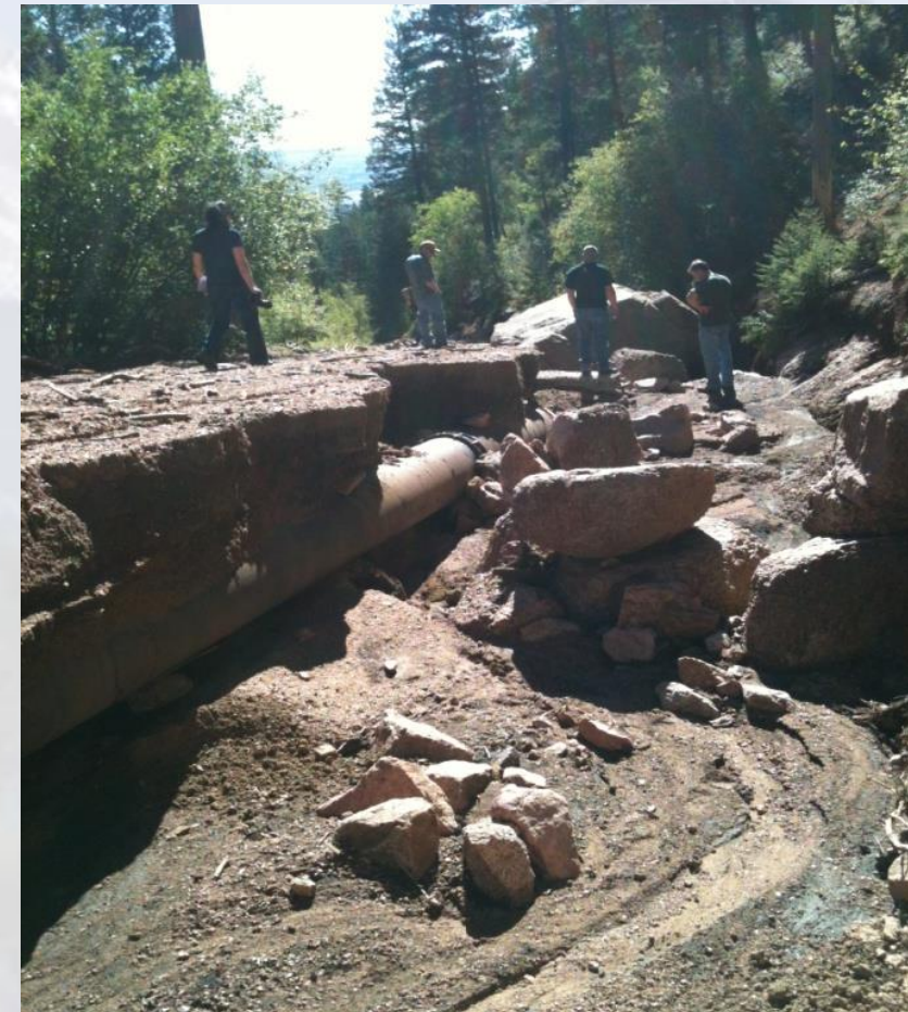
Post Waldo Damage
