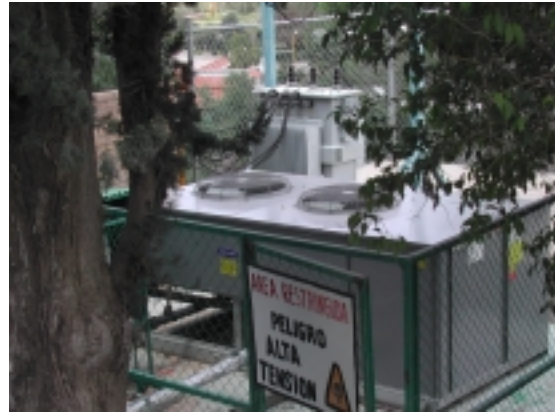
Figure 10. Chiller, Hotel Camino Real
