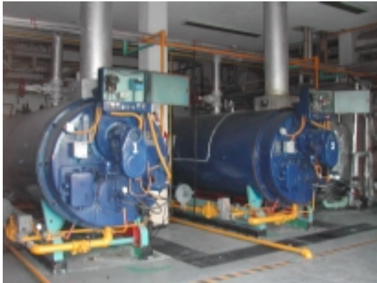
Figure 9. Boiler Room, Hotel Camino Real
