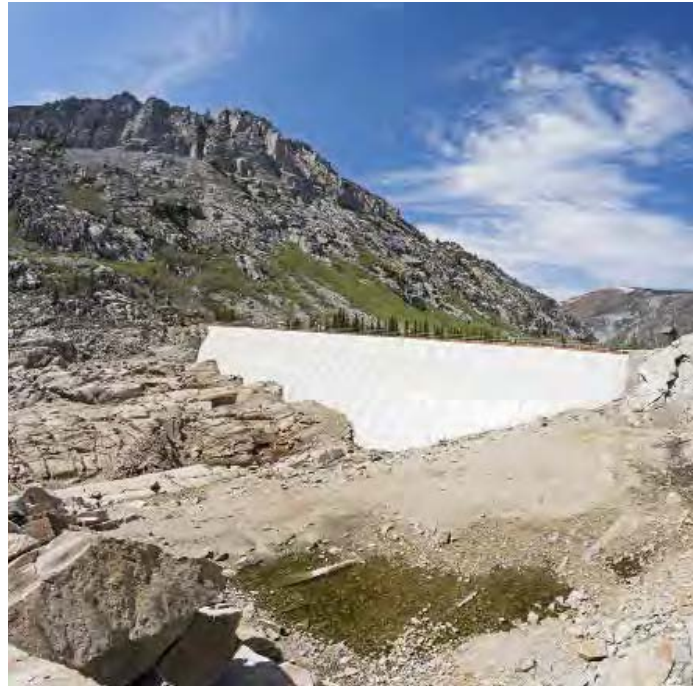
The South Lake Dam in California’s Sierra Nevada shows signs of drought conditions affecting many states in the west.
